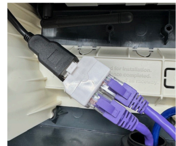
Ethernet cable to AC Coupled inverter
